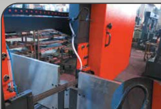
33- PROXIMITY SWITCH FOR SENSING BLADE SLIPPAGE
